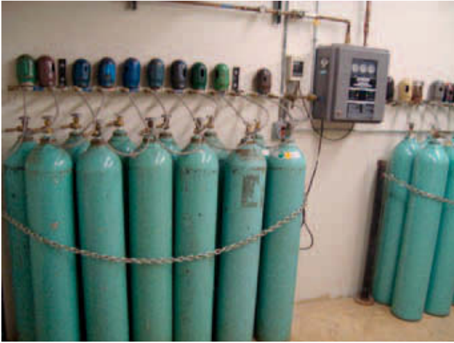
Figure 14-14 Manifold connecting a series of N 2 O and O 2 cylinders for use in a central system. Manifold provides automatic switch over from the cylinder in use. (Courtesy James Soler.)
