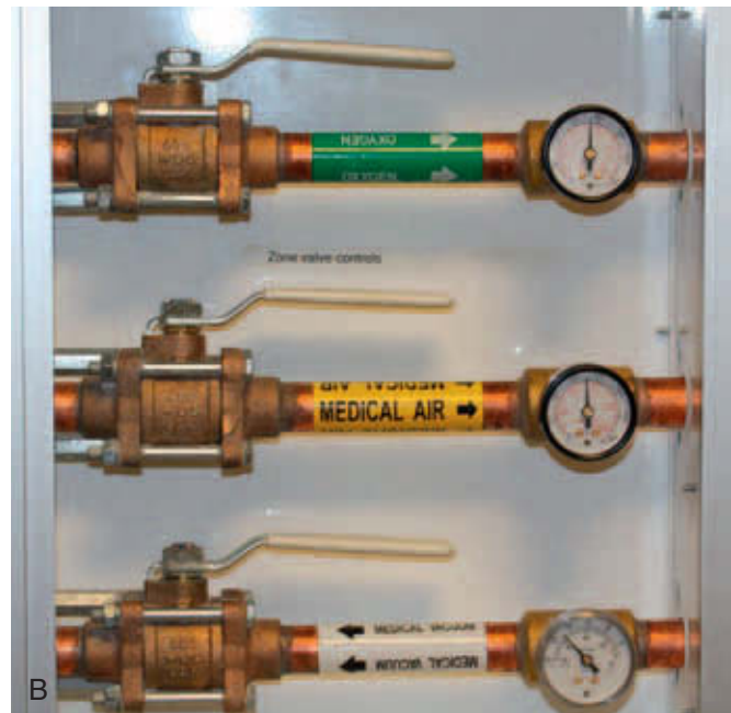
Figure 14-35 A , Alarm system for central system. Alarm is activated when O 2 or N 2 O pressures are low or high and when reserve tanks are in use. B , Central medical gas valve shutoff.
